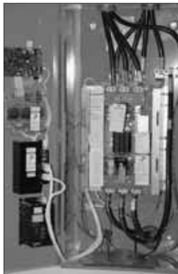
This transfer switch activates standby power for the computer room as needed. Roman installed battery-powered UPS systems for immediate backup power and a 250 KW diesel generator for up to 24 hours of standby power.
