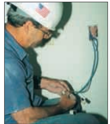
Al LeRay, Roman TechNet communication technician, installs a data jack for category 5 cable which can be used for both telephone and computer networks.
